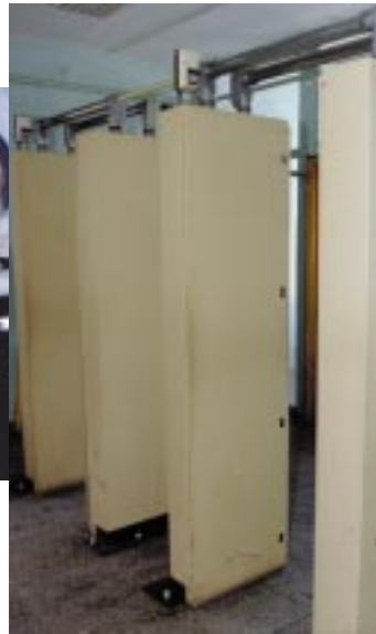
Figure 7. Portal monitors installed by MPC&A program in Russia
