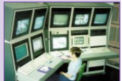
New Central Alarm Display Console in Kiev, Ukraine
