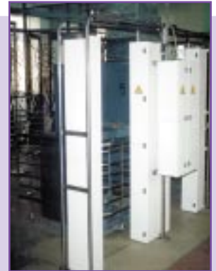
Pedestrian Portal Monitor at Tomsk-7 Enrichment Plant
