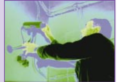
Video Monitor Installation
